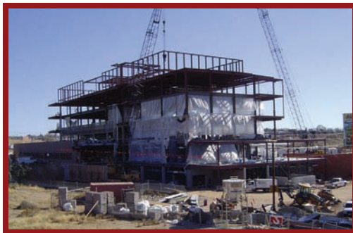
Above: Tri-Lab building site at I-25 Frontage Road north of Mountain Road.
